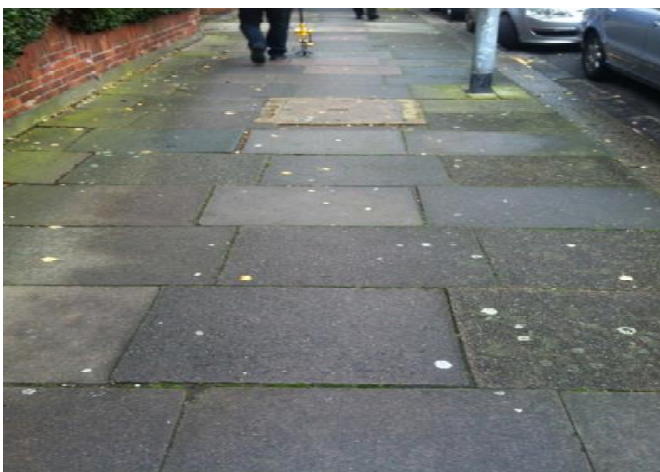
BEFORE: Stamford Brook pavement
