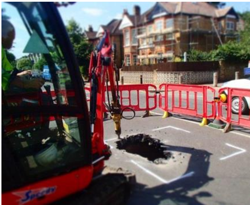
The hole was caused by a collapsed sewer more than five metres underground.
