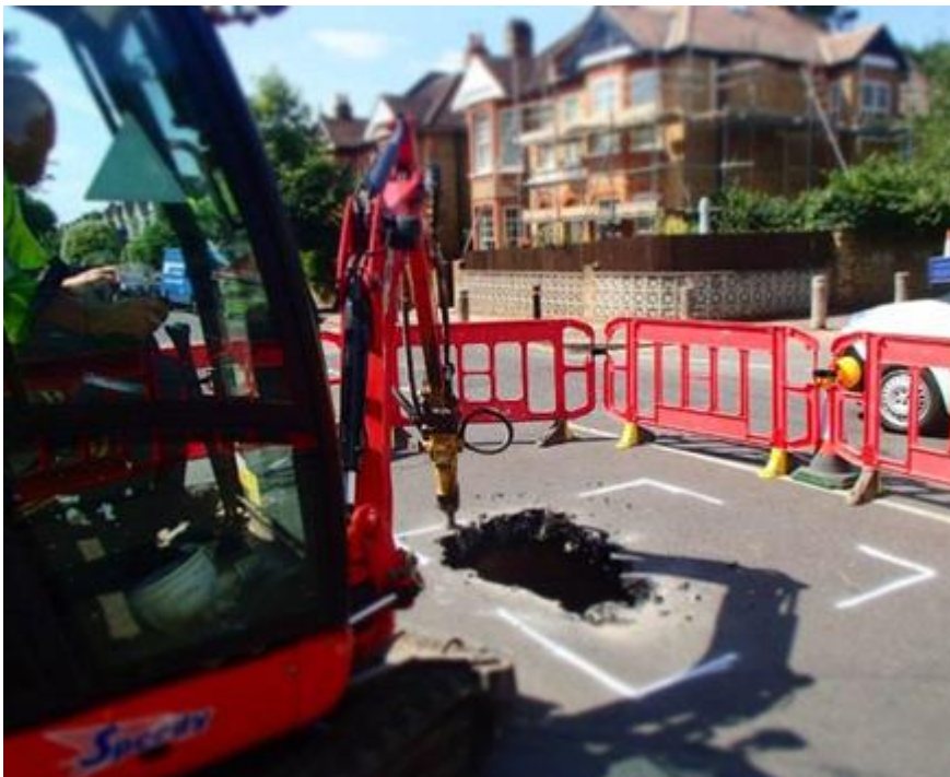
The hole was caused by a collapsed sewer more than five metres underground.
