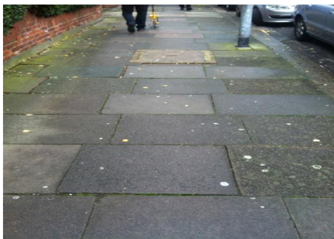
BEFORE: Stamford Brook pavement
